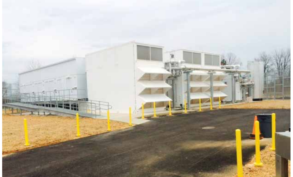
MARCC Data Center at the Johns Hopkins Bayview Campus in Baltimore, MD
